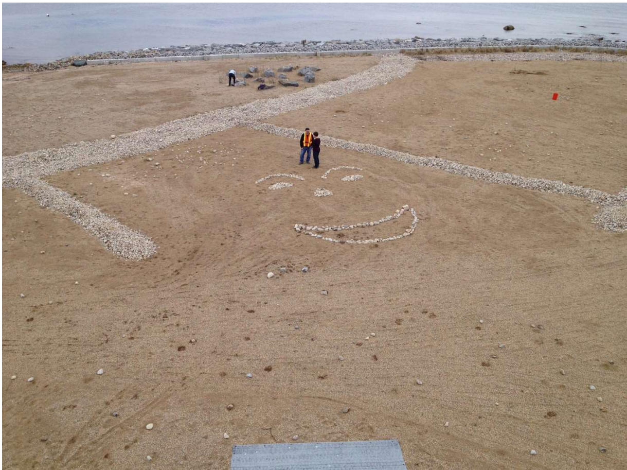
Figure 34: Bird Island, Massachusetts, April 2018. Island has been newly capped with coarse fill and drainage channels have been expanded and augmented. Cobbles have been distributed across the new fill to provide the surface heterogeneity that appeals to terns. C Mostello. MassWildlife
